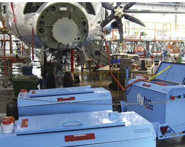
Coolspool 580: Q400 – supplying power during heavy maintenance
